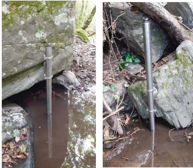
Fig. 1: Sensor installations in brooks with steel pipes and anchored to rock blocks. October 2021.
