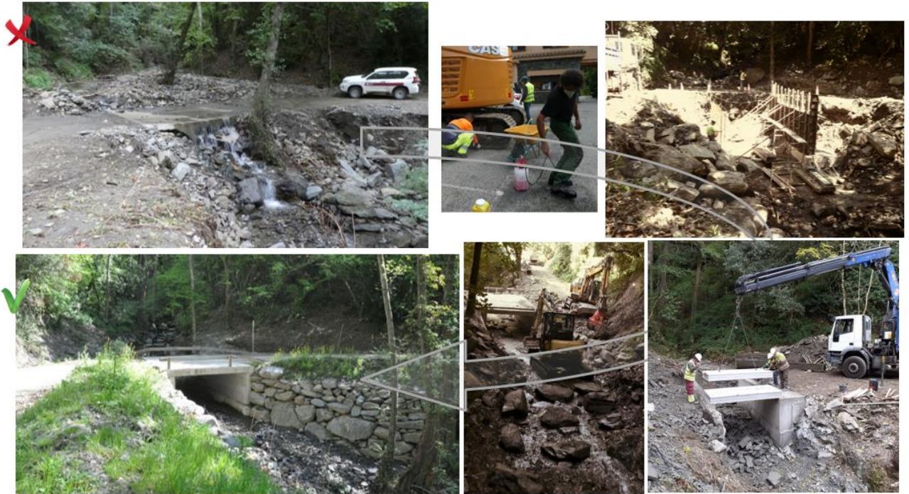
Process of disinfection of equipment, removal of drainage pipes, recovery of the stream bed and construction of the bridge.
